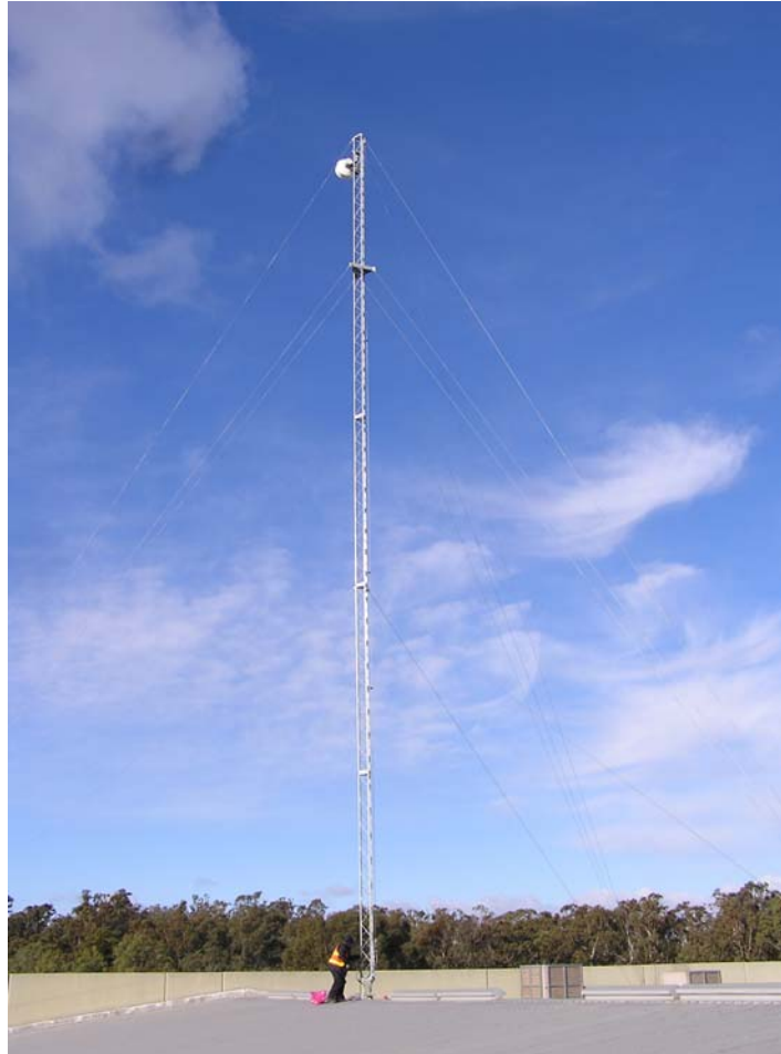
25m mast at SPCA facilities at Mooropana
