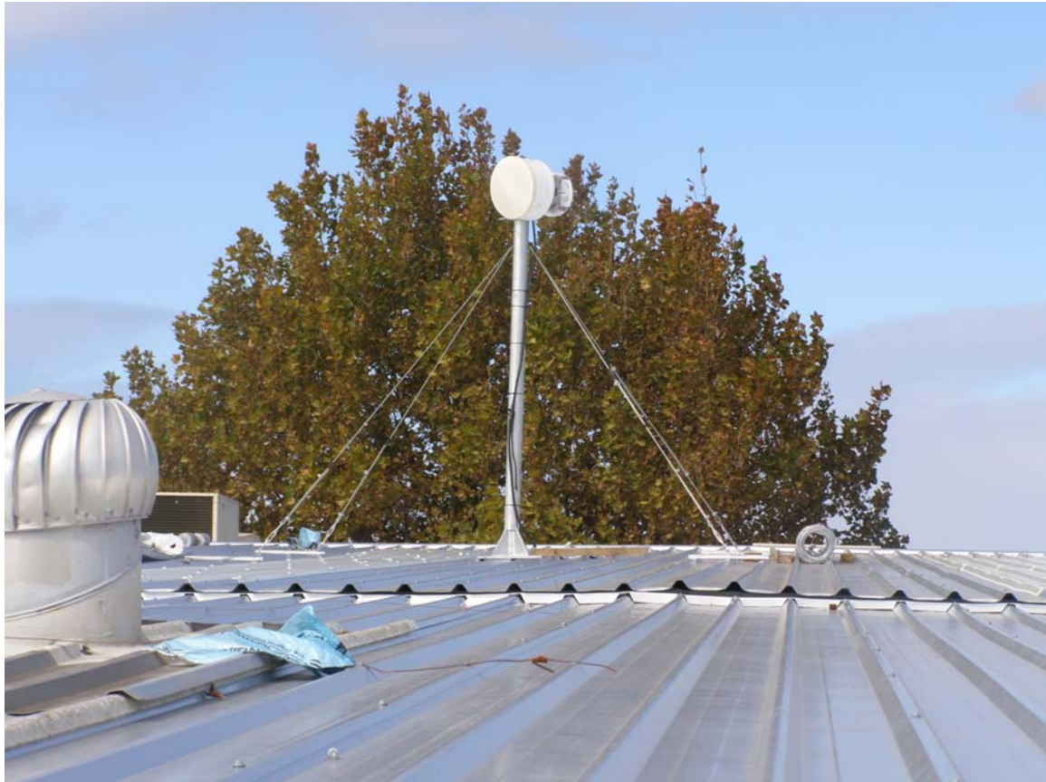
Wave1's MV400 Licensed Microwave on the SOS Print & Media Warehousing Facility
