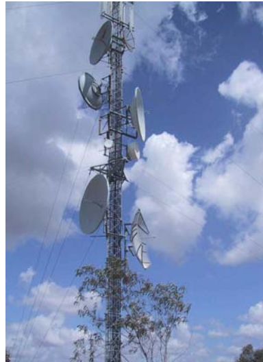
Repeater site with 2 x Macarthur Coal antennas
