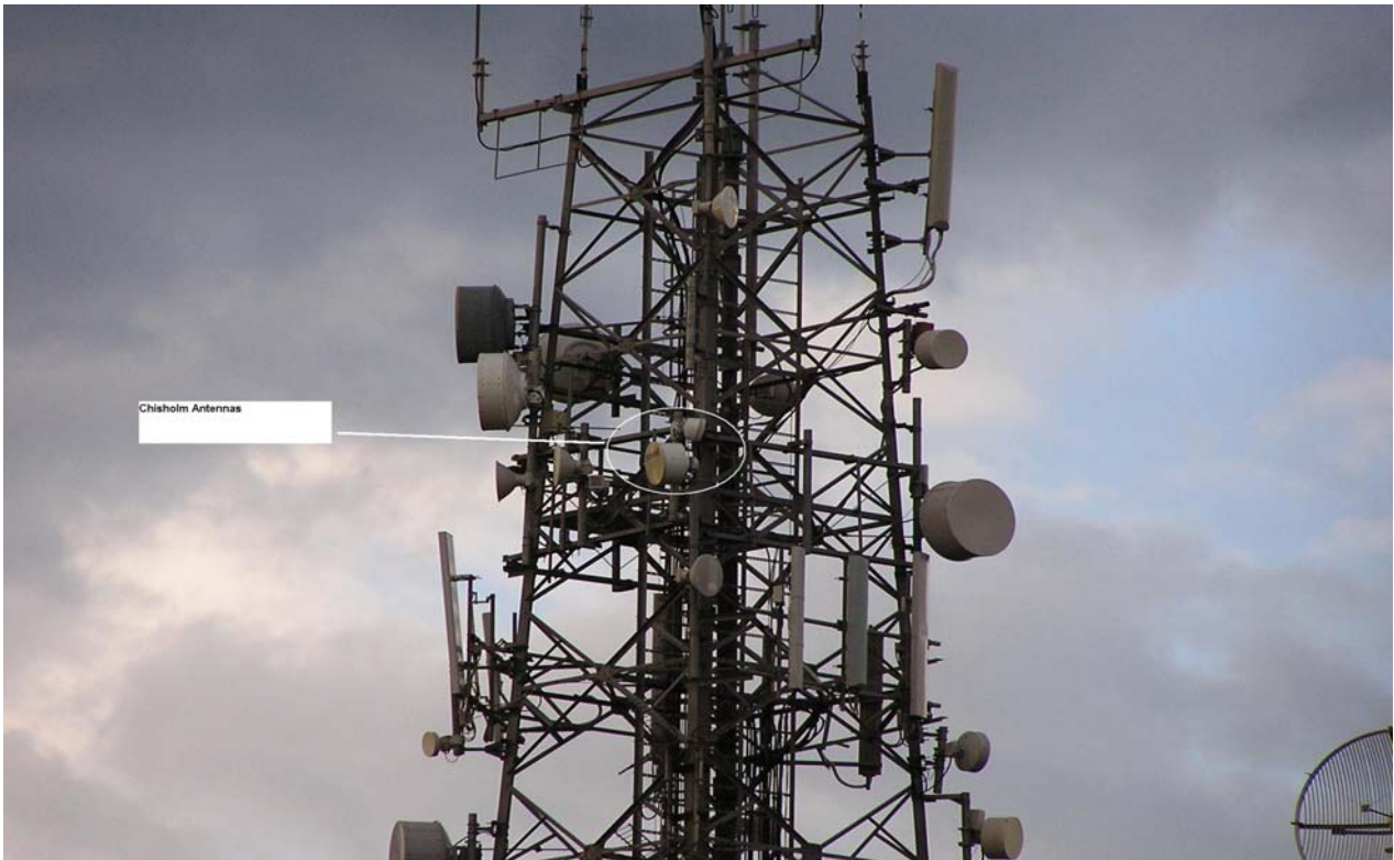
Chisholm Microwave Antennas on Crown Castle Tower installed at 40 Meter height
